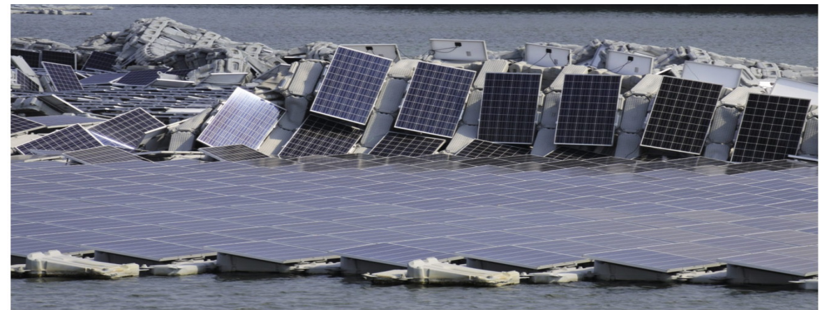
After the outermost row had ripped off the wind-facing edge did not have any ballast anymore to counter uplift from wind. The modules and floaters began to curl-up with the result of an electrical fire.
