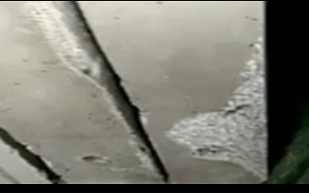
Joint Crack and Peel Off
