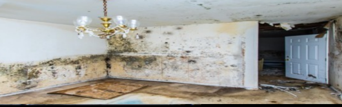
Mold and Fungus
